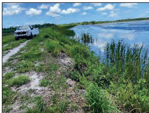
Photo 16 - North Reservoir. Sparse Vegetation and Early Erosion Area Near Center of North Levee.
