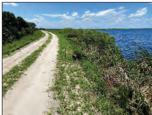
Photo 5 - South Reservoir. Sparse Vegetation and Early Erosion Area on East Portion of South Levee.
